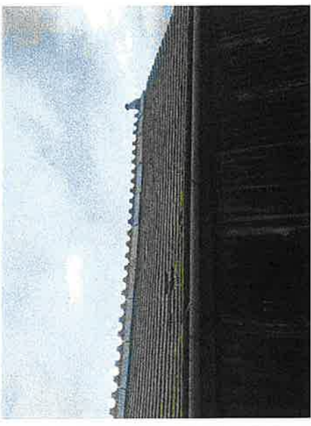
Lifted, missing and slipped roof tiles
